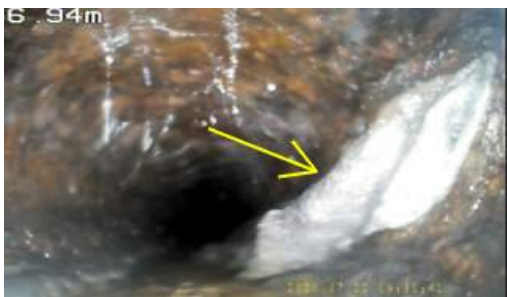
Photo 3-1 looks like a rag or towel of some sort. Recommend Cleaning line
